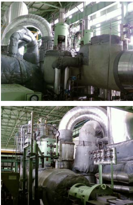
Fig. 1 Turbine main stop valve and control area on a thermal electric power plant.
