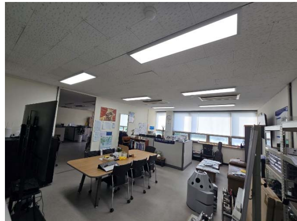
Fig. 2. Flat-panel LED lighting installed office.
