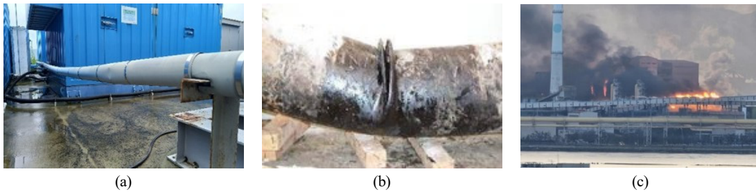
Fig. 1. Accident Cases in Non-conventional Oil Pipelines: (a) Buckling Deformation of Yeoncheon Oil Pipeline, (b) Oil Pipeline Destroyed due to Buckling, (c) POSCO Factory Fire Accident
