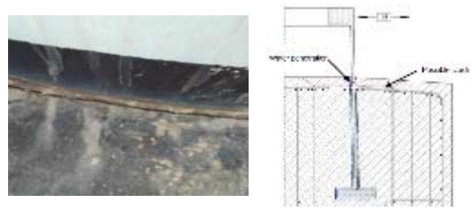
Fig. 1 Damages within the transition areas [5, 6]
