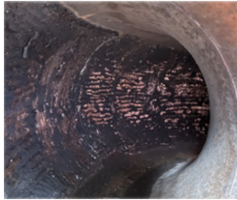
Fig. 3. Example of wear of bend pipe
