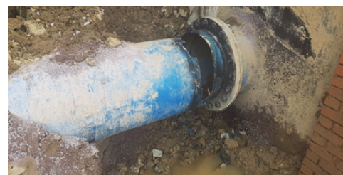
(a) Damaged pipeline at valve chamber
