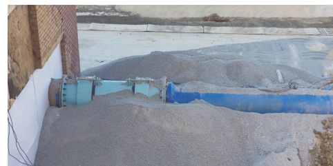
(b) Installed expansion bellows
