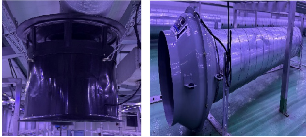
Fig. 1. Appearance of installed convection fan (left : vertical convection fan, right : horizontal convection fan).
