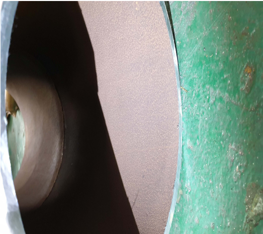
Fig. 1. Metal Particle in Oxygen pipe
