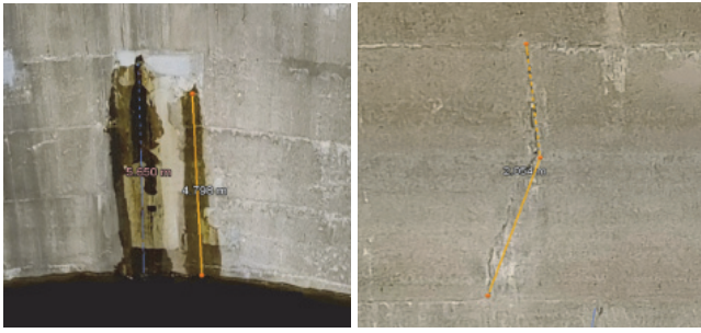
Fig. 6 Detailed Damage Identification of YCN Dam Spillway
