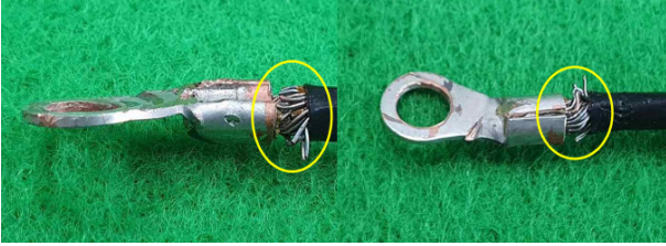
Fig. 5. Inappropriate case of crimp terminal of chiller heater connection.
