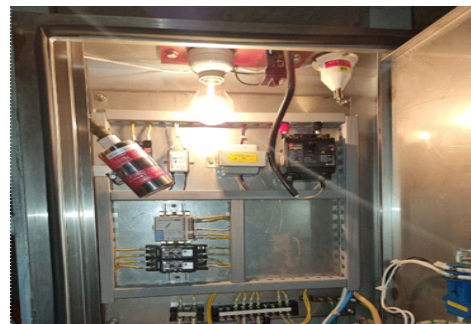
Fig. 2. Inside the light control panel
