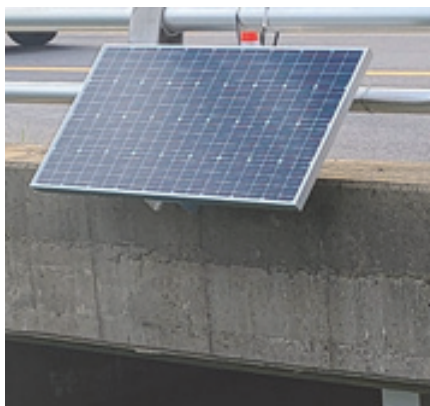
(a) Solar panels
