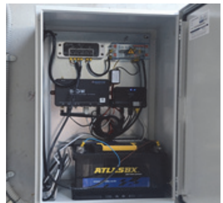
(c) Network equipments
