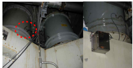
Fig. 1 Vibration monitoring location of cooling fan of reactor containment building at ANO. (10)
