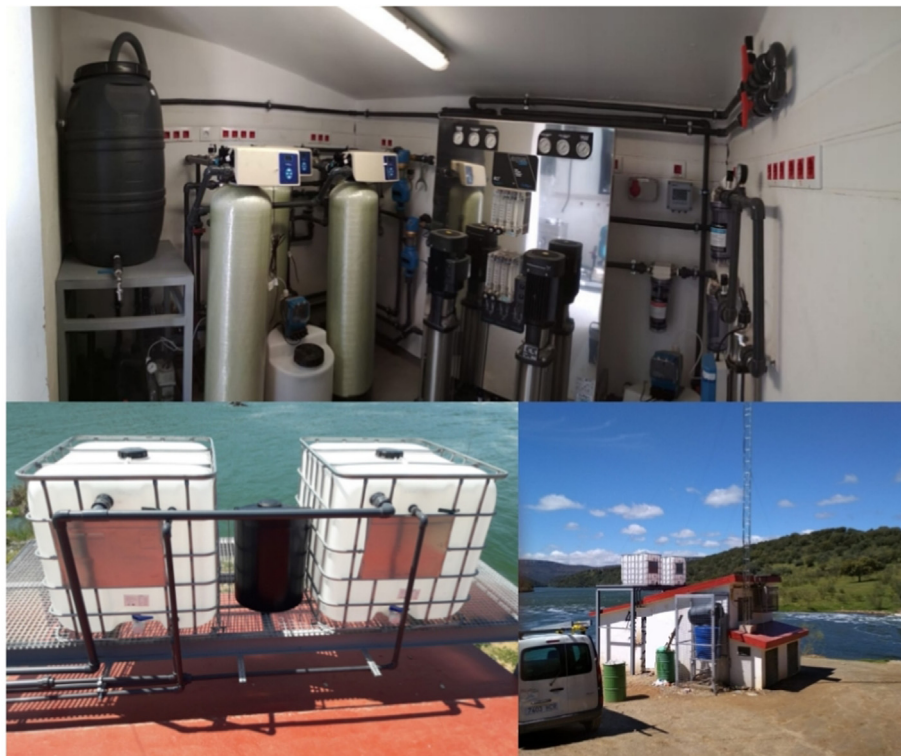
Fig. 4. Above: Picture of the water treatment plant. Below left: 1 m 3 water storage tanks for rejected and pure water. Below right: Arrocampo water discharge monitoring station.
