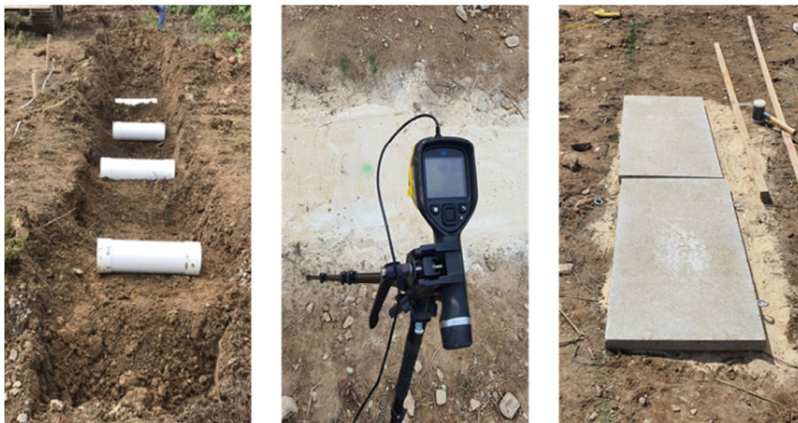
Fig. 5. Experimental conditions for obtaining thermal image: (a) schematic drawing of field test; (b) photograph of installed cavity
