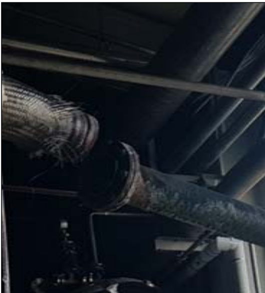
Fig. 2. Flexible hose destroyed by accident.
