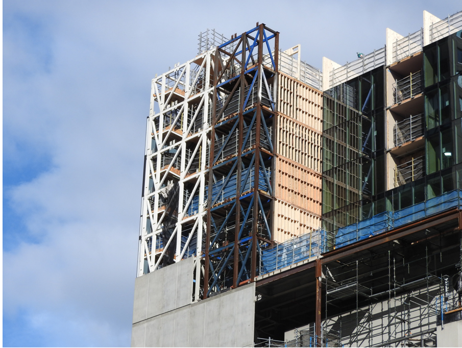
Figure 3. Hybrid multi-storey construction, combining steel framing, precast concrete and EWS. (Source: G. Marfella)
