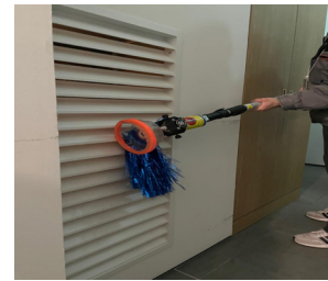
③ Check whether the blower is working
