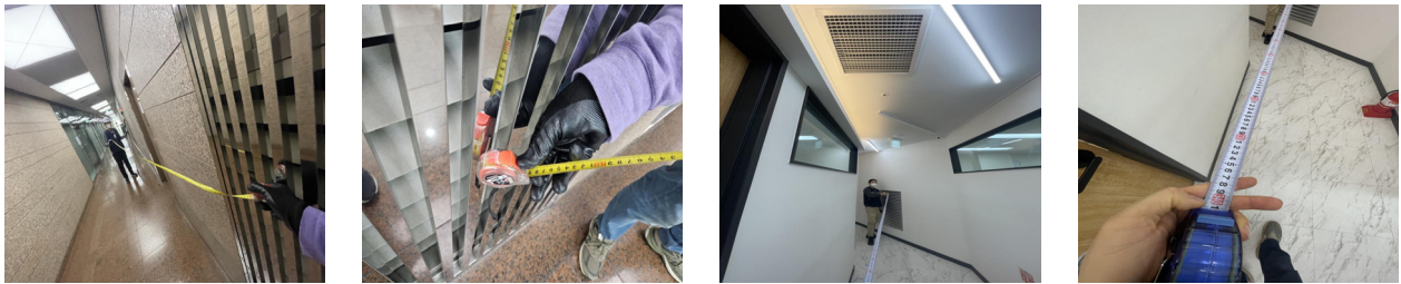
① A firefighting object at a business facility located in Gangnam-gu, Seoul. As a result of measuring the distance between the lower supply air ~ the upper exhaust duct, 2.89m
