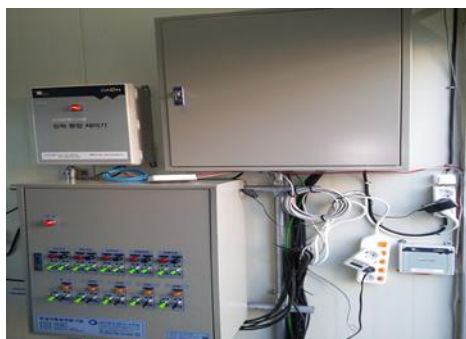
Figure 1. House control device wind direction, wind speed, precipitation
