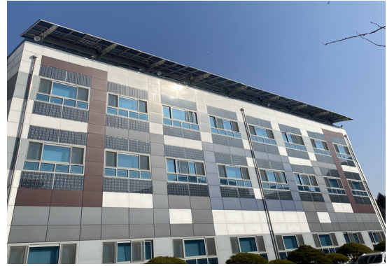
Fig. 1. BIPV system applied building
