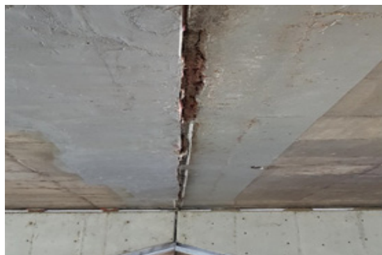
(c) Re-damage in Deck Slab
