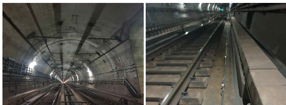
(a) Photographs of tunnel convergence meter sensor installation (b) Photographs of STL sensor installation
