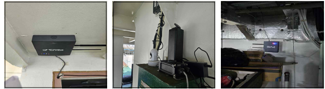
Fig. 4 Installation in Living Lab Site (Passenger Ship)
