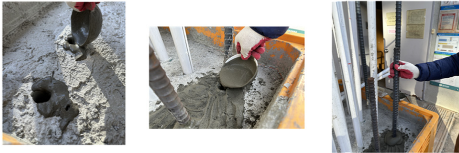
(a) Installation of deformed rebar after filling the cement mortar into a drill hole
