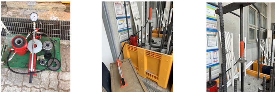
(c) Insertion of the incised steel pipe into a drill hole using hydraulics and reaction beam
