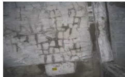
(a) Micro cracks
