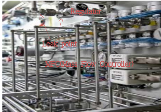
Fig. 2. Plasma Chemical Vapor Deposition (PCVD) Gas cabinet interior configuration.
