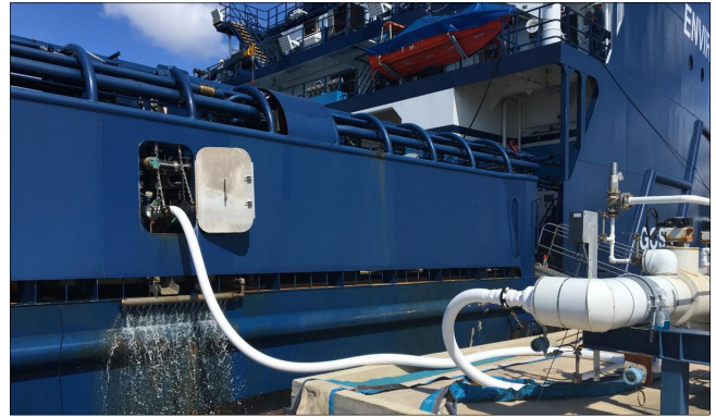
Fig. 6. Pipe to ship LNG Bunkering. (Source: Trelleborg, 2018)
