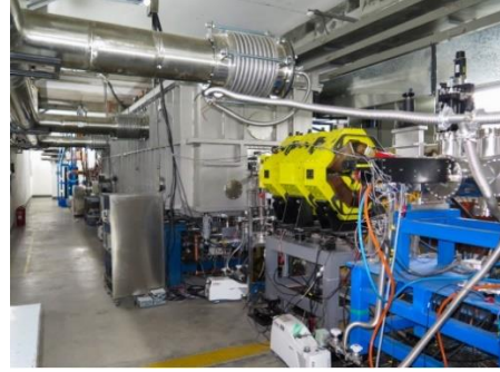
Fig. 9. HCM6 and transfer lines in tunnel
