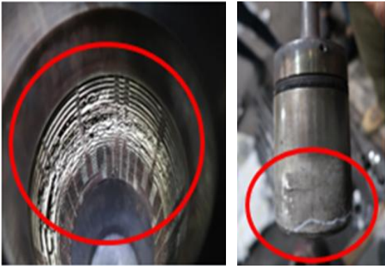
Fig. 1 Control valve cage and plug damage
