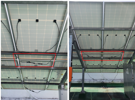
Fig. 3. Simulated Voltage mismatch using MC4 cable
