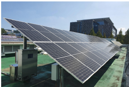
Fig. 1. 10 kW PV System in KIER
