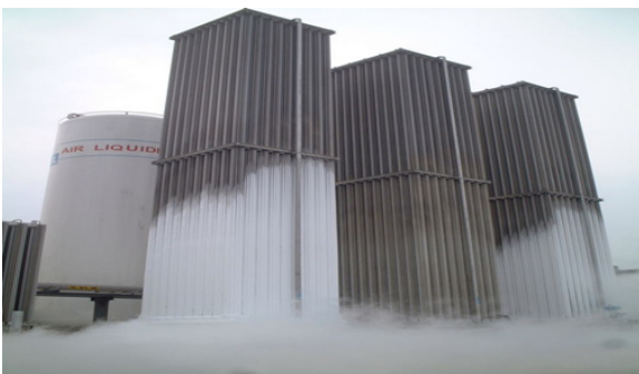
Fig. 3 Fog and frost generated during AAV operation
