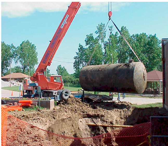
Fig. 1. Underground emergency fuel tank.
