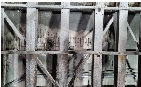
Fig. 13. The case of 2 arch tunnel (Fracture of center wall)
