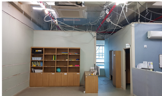
(a) Lack of upper cable management
