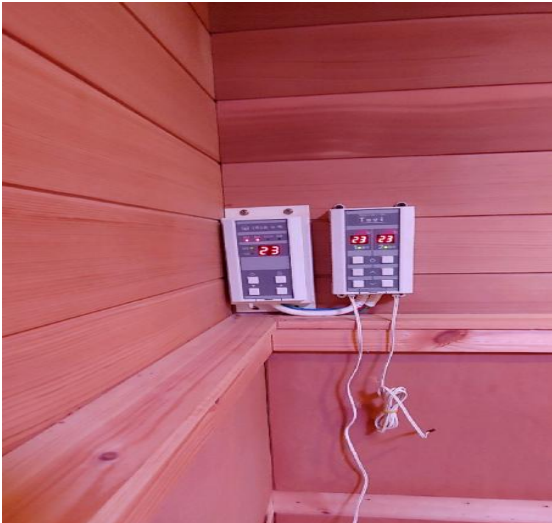
Fig. 5 Air temperature controller and temperature sensors inside container house
