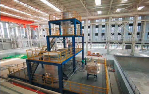
Fig. 3. Integrated safety system verification and test bench of multipurpose small PWR.
