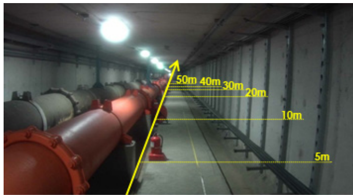
Fig. 3. CCTV visibility range in the underground utility tunnel
