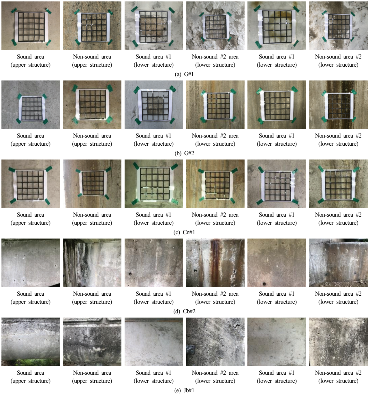
Fig. 1. Surface rebound value measurement area on concrete bridges (part of the measured value)
