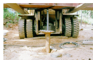
Fig. 6. Rock-grout bond failure (Highly weathered, depth =1.0m)
