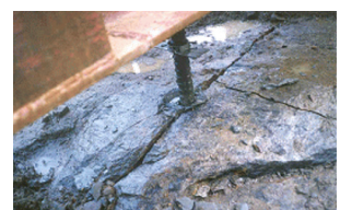
Fig. 7. Rock failure (Moderately weathered, depth=2.0m)
