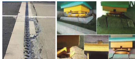
Fig. 1 Daegu-Pohang expressway damage case[1]
