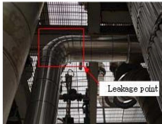
Fig. 2. Leakage point of accident site.
