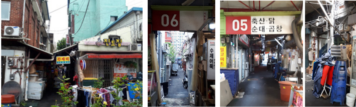
Fig. 3. Deteriorated Residential Facilities and narrow alley with combustible materials
