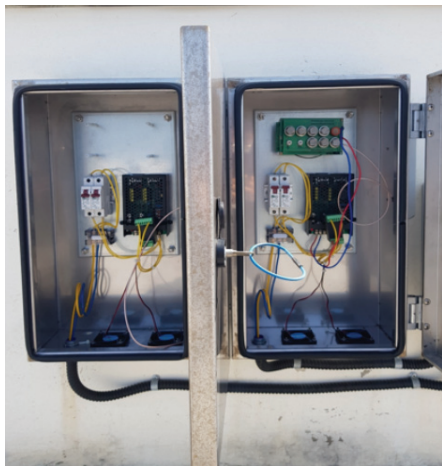
(a) Installed sensor box
