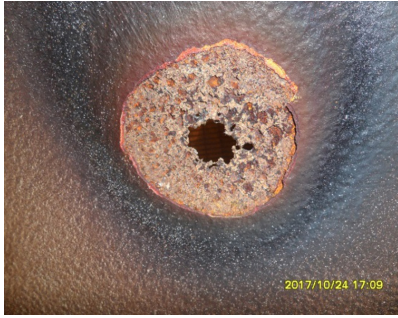
Fig. 4 Damaged inside surface.
