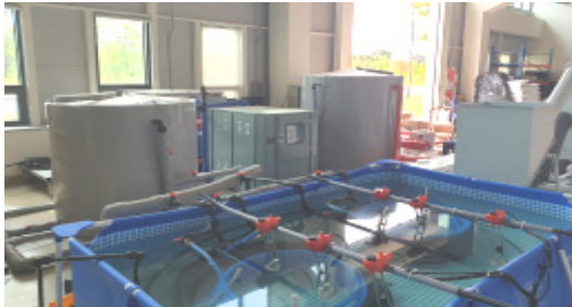
Fig. 1. Experimental waste heat recovery system
