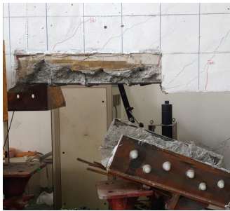
(a) Anchor Failure
