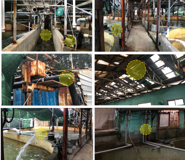
Fig. 2. Deeteriorated fish-farm site
