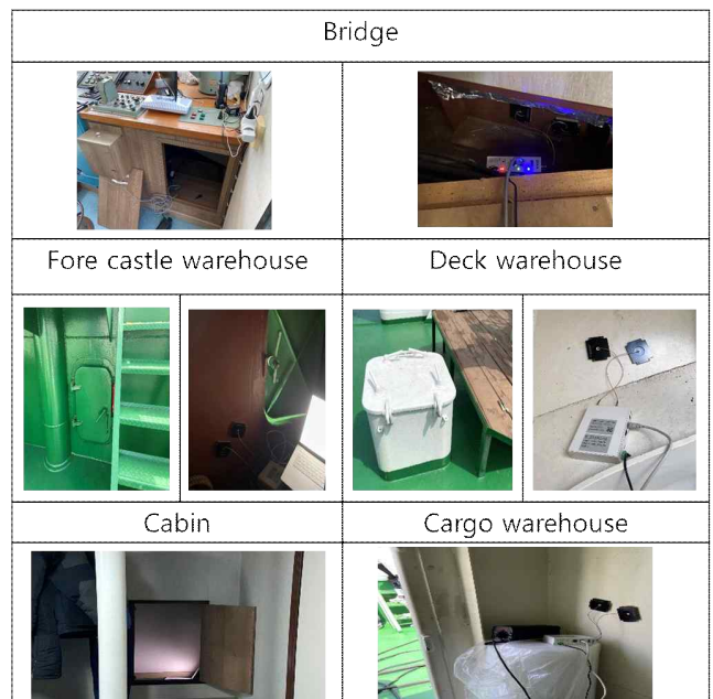
Fig. 11 Detailed installation of each point of surface wave generator for speed test
