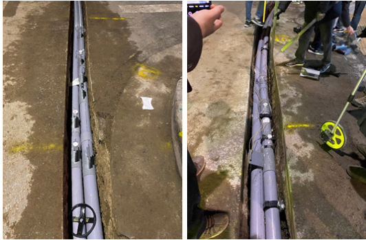
Fig. 6. Sensor installation on Seoul Yang-cheon district
