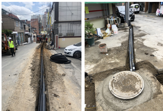
Fig. 2. Sensor installation on Busan Yeon-je district
