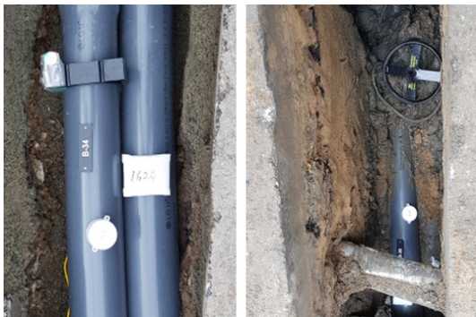
Fig. 4. Limited installation on Busan Yeon-je district
