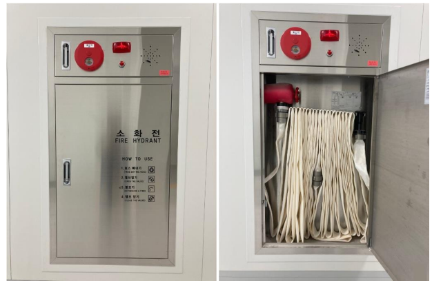
[Figure 1] Rack-type Fire Hose
